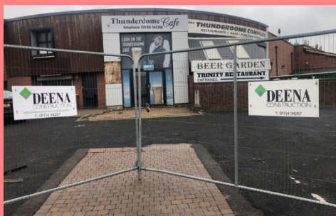
Figure 32: Example of Thunderdome Cafe vacant site in town
